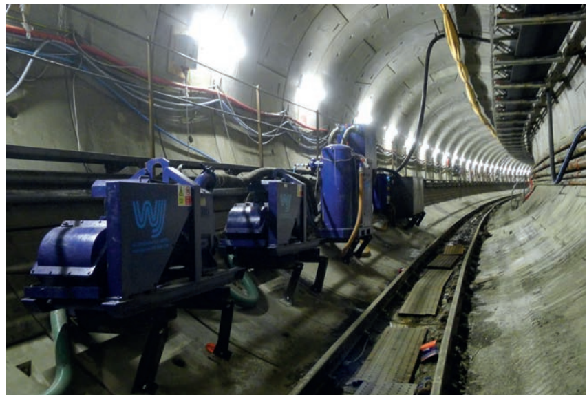
Above: Figure 4, In-tunnel wellpoint system used for active pumping of wells for cross passage construction PHOTO COURTESY OF WJ GROUNDWATER LIMITED
