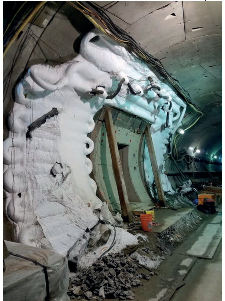
Above: Figure 3, Artificial ground freezing used in cross passage construction PHOTO COURTESY OF SOILFREEZE INC
